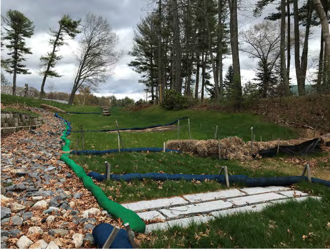
Fig 9: Slope above the manhole at Gundalow Landing/east side of the bay. Viewing east. (04-30-21)
