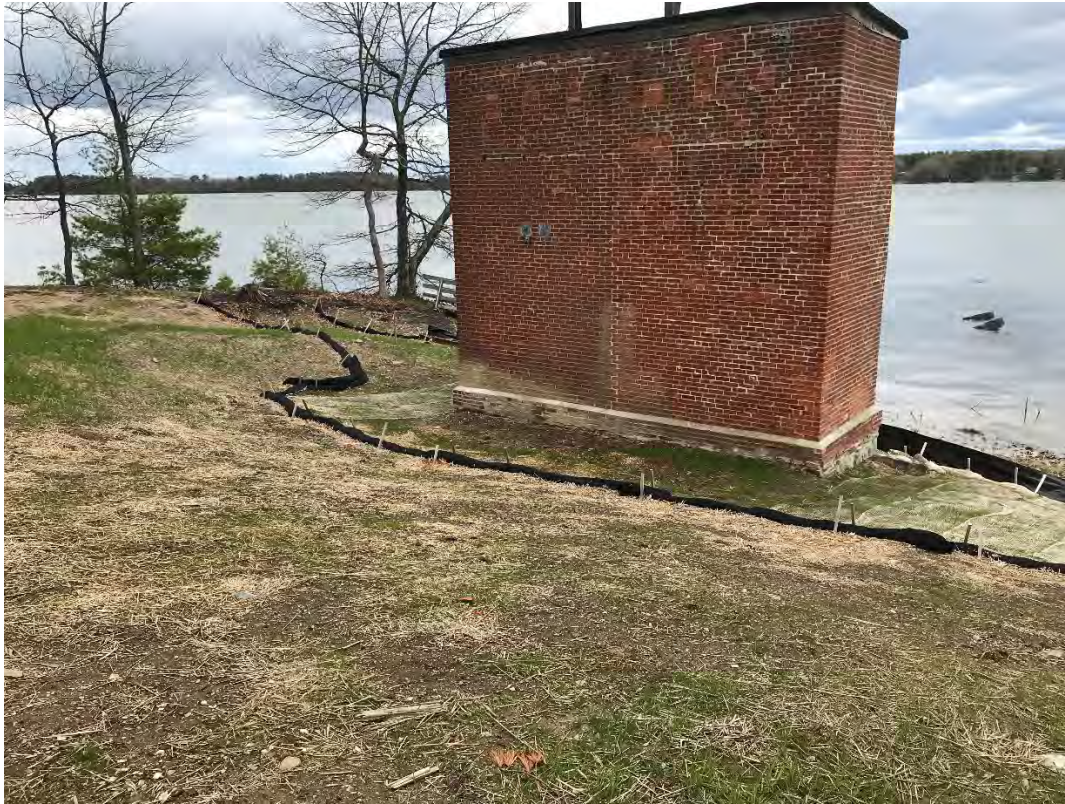
Fig 1: Slope leading down to cable house and salt marsh restoration at the west side of the bay. Viewing northeast. (04-30-21)
