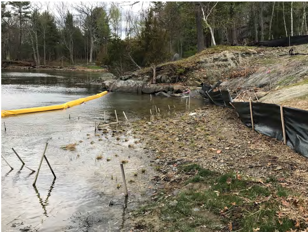
Fig 4: Toe of the slope and salt marsh restoration at the west side of the bay. Viewing south. (04-30-21)
