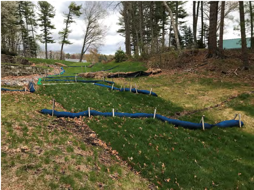
Fig 10: Slope below the manhole at Gundalow Landing/east side of the bay. Viewing east. (04-30-21)
